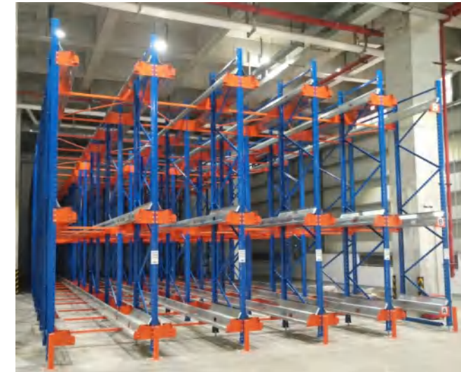
Radio shuttle rack project 穿梭式货架案例
