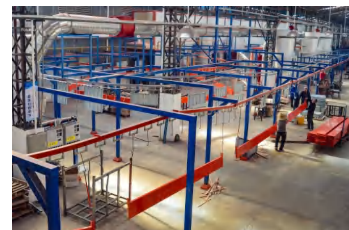
Painting line 喷涂线
